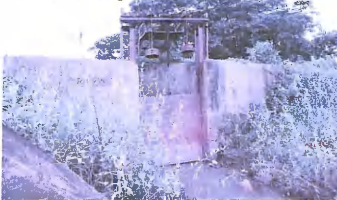
An Abandoned Irrigation Sluice Gate at Borkola Village
